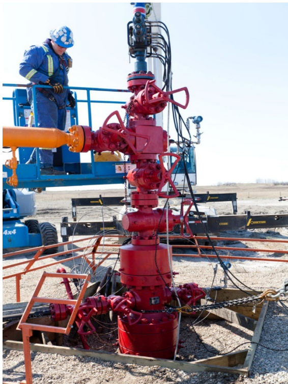
Figure 1. Current Aquistore injection well.
